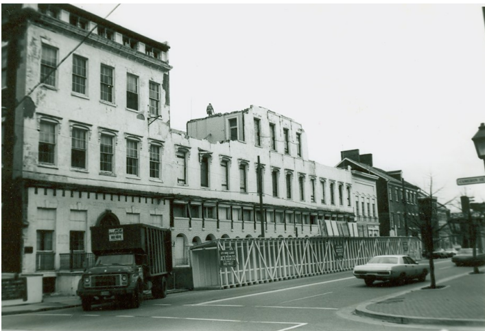
The Carlyle Apartments from Fairfax St and Cameron St, under demolition in 1972. Property of Carlyle House Historic Park.
