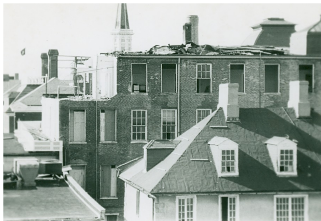
The Carlyle Apartments, under demolition, and the Carlyle House pictured from Lee St. Property of Carlyle House Historic Park
